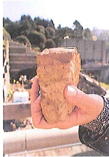
An example of the crumbly rock miners are encountering on the west side of the tunnel. Photos: Karl Nielsen
