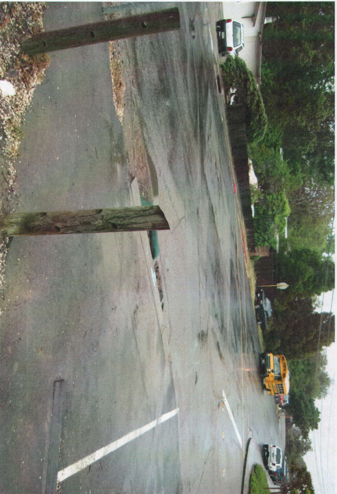
A UNIMPROVED CORNER OF SAN JUAN AVE AND ALVARADO AVE PROPOSED TO BE IMPROVED WITH ADA CURB RAMPS AND SIDEWALK.
