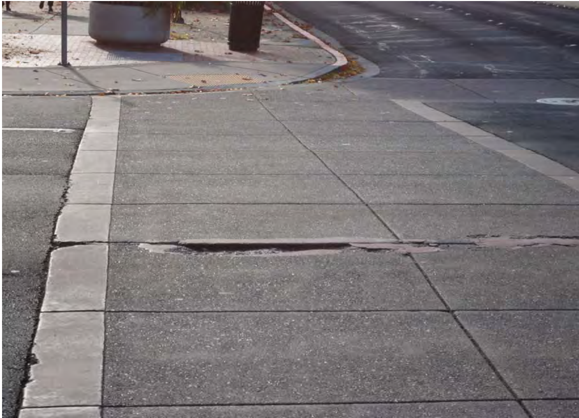
7. Clayton Road @ Grant St: Proposed improvements include replacing existing pothole & crack-ridden crosswalks with ADA-compliant, high-visibility color concrete crosswalks.
